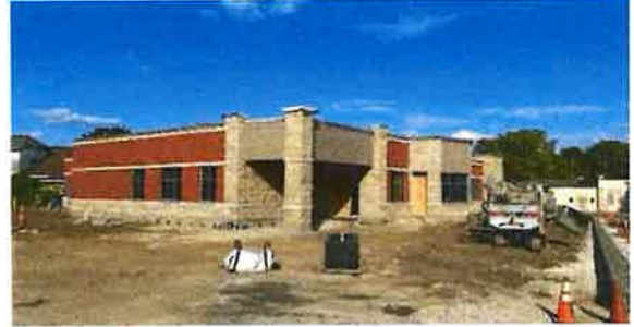
View of the exterior from the construction entrance at the southwest corner of the site, looking northeast.
