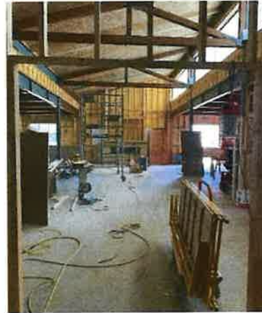
View in the clerestory, looking east towards the fireplace. The translucent panel and fireplace stone are in place.
