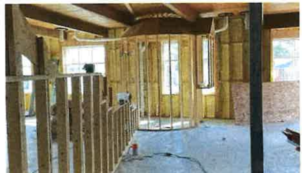
View, looking south, of the wall between youth and adult with the silo at the end of the wall.
