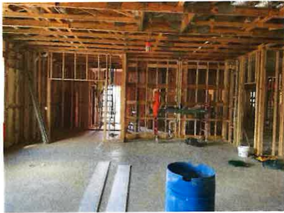
View of Meeting Room 102, looking north to the storage room and kitchenette.
