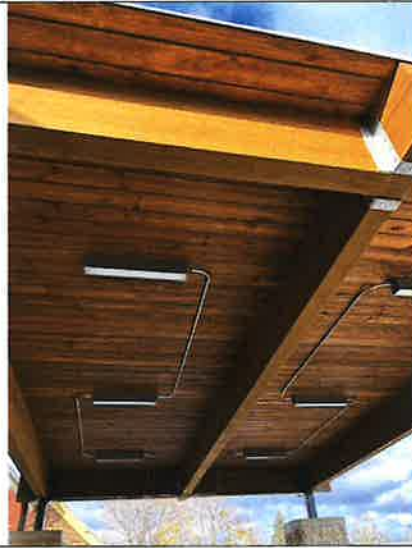
View of the shade structure lighting. To be rotated.
