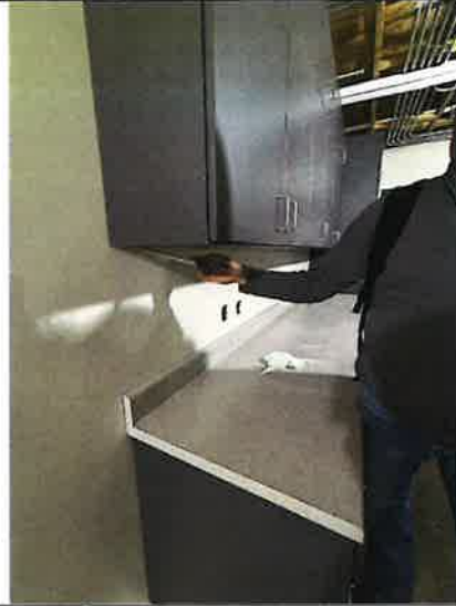
Staff workroom casework – under cabinet lighting
