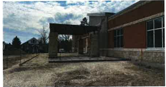
View of the exterior from the north of the site, looking south at the patio slab.
