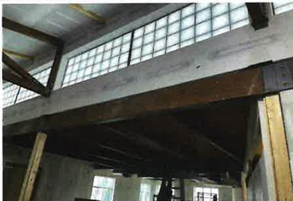
View of the clerestory framing and the glulam infill at the steel beam. Exposed steel is to be painted.
