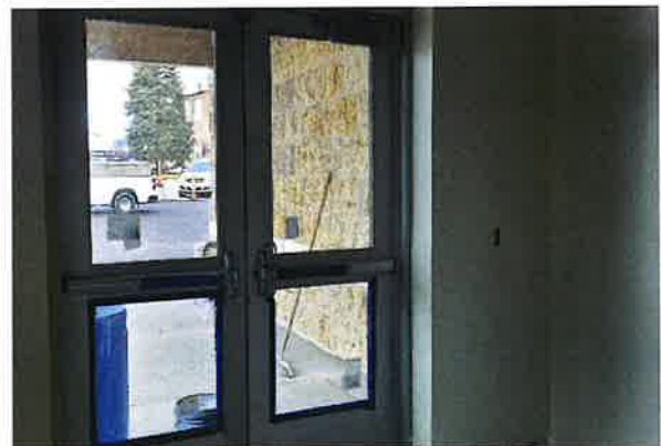
View of the front entrance showing the door that will require the ADA operator to be moved and door replaced.
