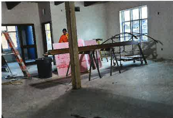
View of the interior showing the majority of the painting and trim being installed.
