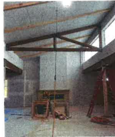
View in the clerestory, looking east towards the fireplace. The translucent panel and wall finish are in place.
