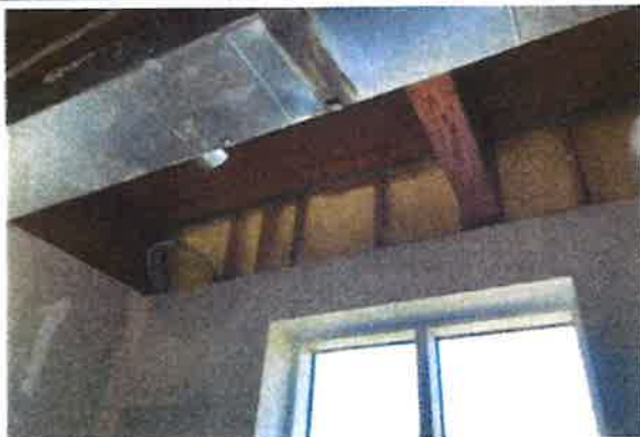
View of at exterior wall with exposed spray foam insulation that will need a thermal barrier.
