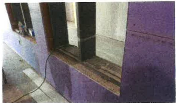
Fire rated window into the corridor that should receive a wood sill, with painted gypsum board head and jamb.
