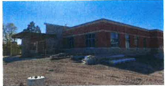
View of the exterior from the northeast corner of the site, looking southwest.
