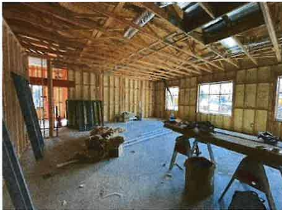
View of Meeting Room 102, looking southwest. Exterior spray foam and windows are installed.
