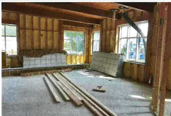
View of Adult Tower Seating 121 with, wood structure, windows, roof drains, and silo edge in the right foreground.
